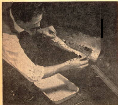
5. Successive layers of Celastic ® may be used to build up spots where the original metal is completely gone. Allow each layer to set 15 to 30 minutes before applying the next one.
